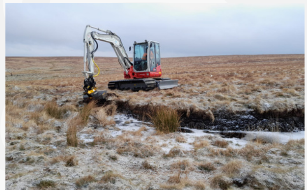
Figure 3 : An example of bare peat at Great Gnats Head, and low-ground pressure machinery carrying out restoration works
