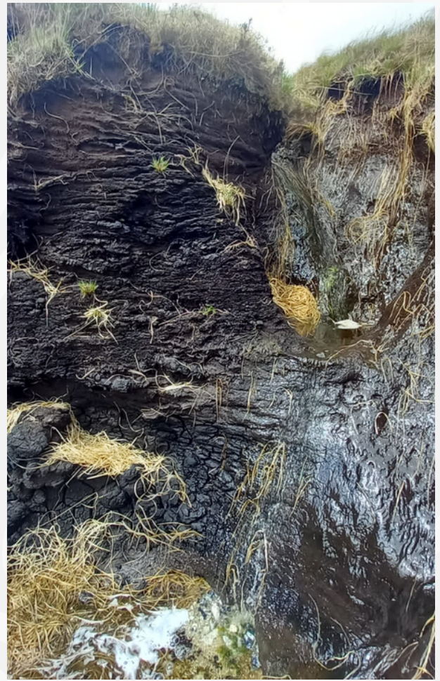
Figure 2 : An example of an eroding gully at Tavy Head. Water can be seen running off the peat, which will be taking peat and dissolved organic carbon away with it. Peat will continue to erode and carbon be lost into the atmosphere and waterways unless works such as reprofiling and blocking gullies take place.
